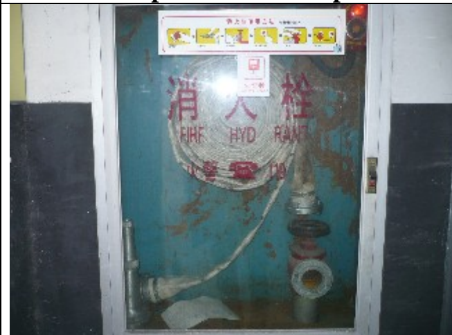
Fire extinguishers and Fire hydrant
