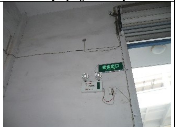
Exit sign and Emergency light
